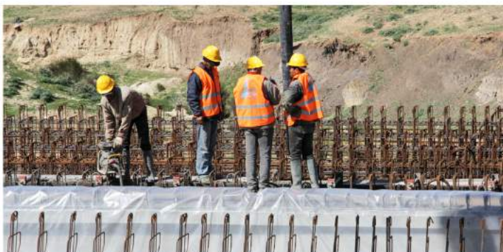
CONSTRUCTION WORK OF A BRIDGE CROSSING OF OUED TESSA ON THE MC60 AT PK75,5 IN THE GOVERNORATE OF KEF.
